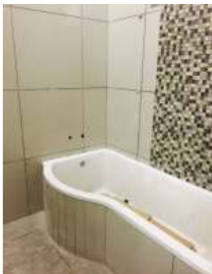
A typical bathroom
